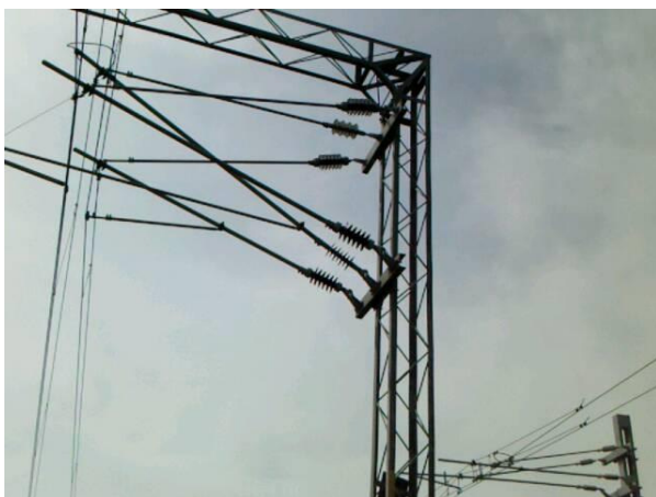
Figure 3: Use of HV insulators for Railway applications; example: 1
