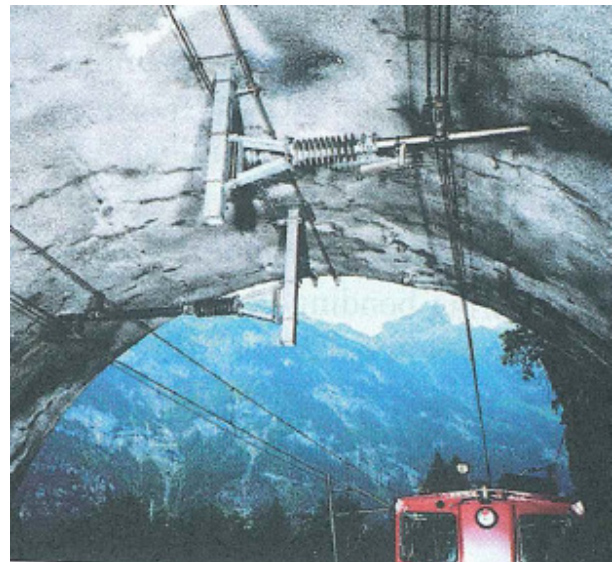
Figure 1: Applications of Composite insulators in European Railways network – Lotschberg tunnel [8]
