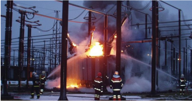
Figure 2: An OIP bushing failure on the 400-kV, 100-MVAR reactor caused this reactor fire [5]
