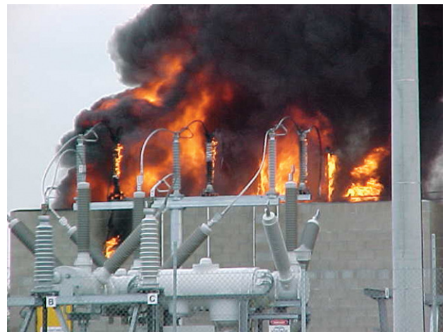
Figure 1: A 110-kV OIP bushing failure caused this 80-MVA transformer fire [5]
